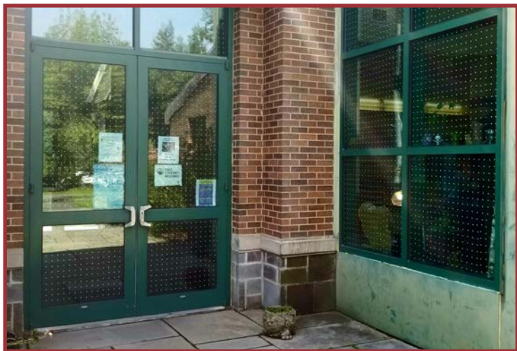
Window dots installed on the windows of the Nature Center.
